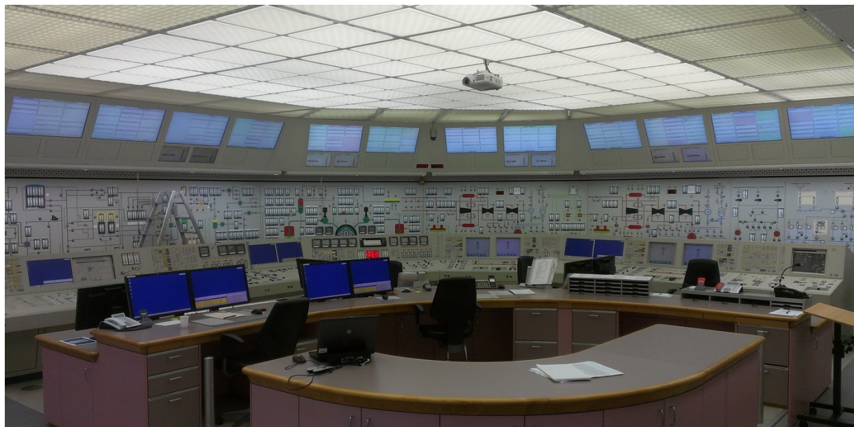
Figure 3 Beznau Simulator Control Room (after)
