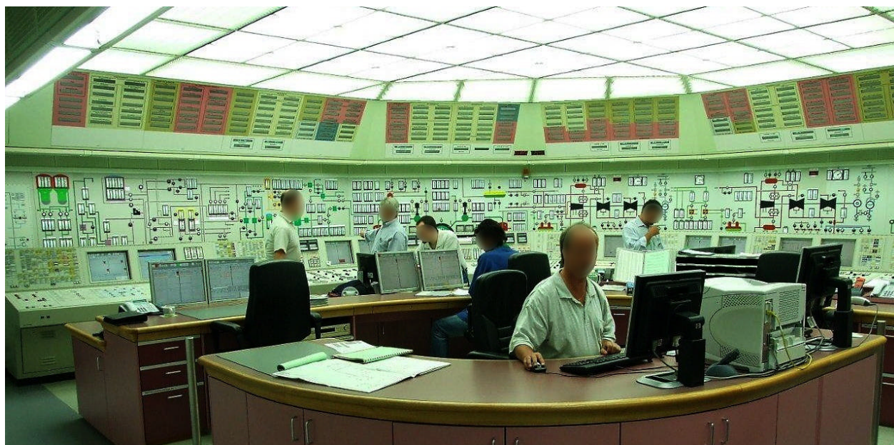
Figure 1 Beznau Unit 2 Control Room (before)
