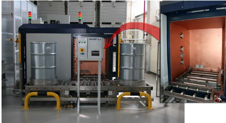
Figure 4 Stationary system for FRM of radioactive waste at Ignalina NPP (Lithuania) and detailed measuring chamber
