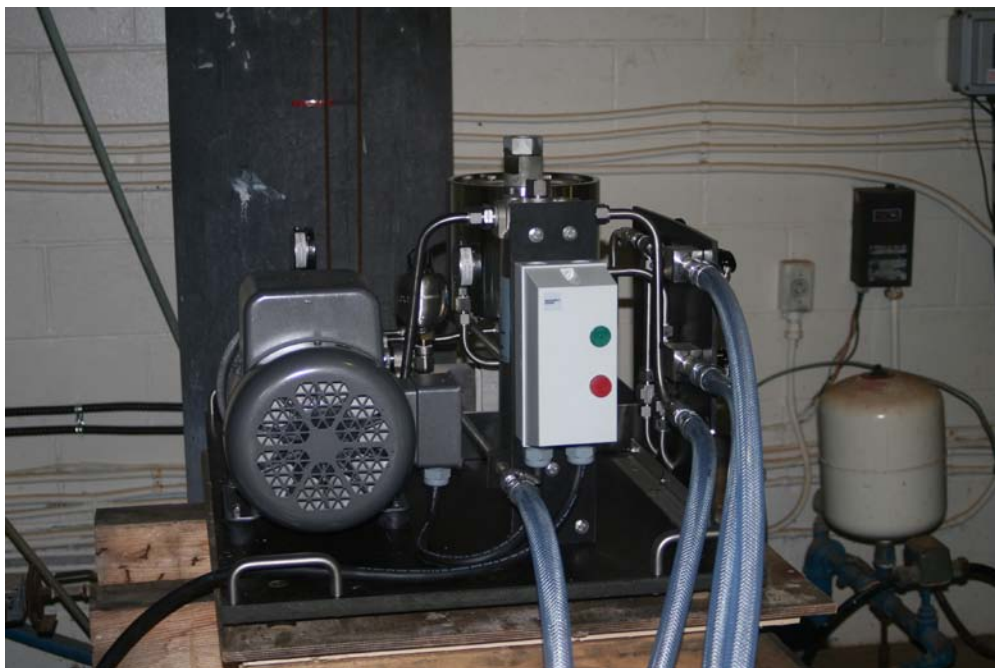
Figure 1. Custom-made Bench Scale RO Unit at Existing Welcome WMF Water Treatment Plant
