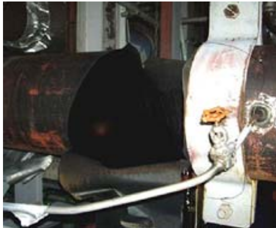
Fig.1 Ruptured Pipe at Mihama-3 [1]
