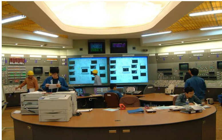
Figure 1 Qinshan CANDU Control Room showing ACCIS Process Displays on Central Projection Screens
