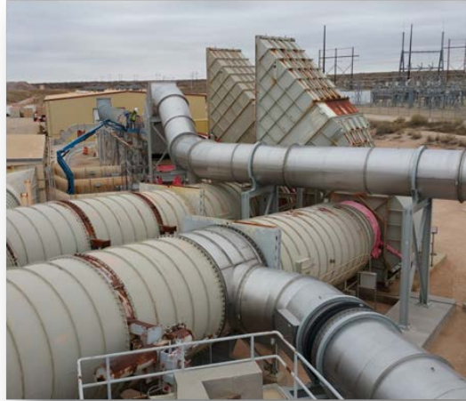
Figure 1. Interim Ventilation System is tied into the Underground Ventilation System to supplement total airflow
