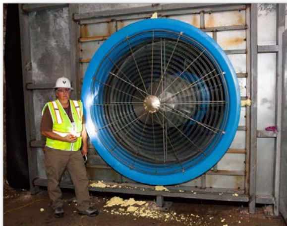
Figure 2. The Supplemental Ventilation System, a fan and additional louvers and baffles to increase airflow through the north part of the mine
