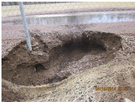
Figure 12 Erosion during wet spring 6 months after installation
