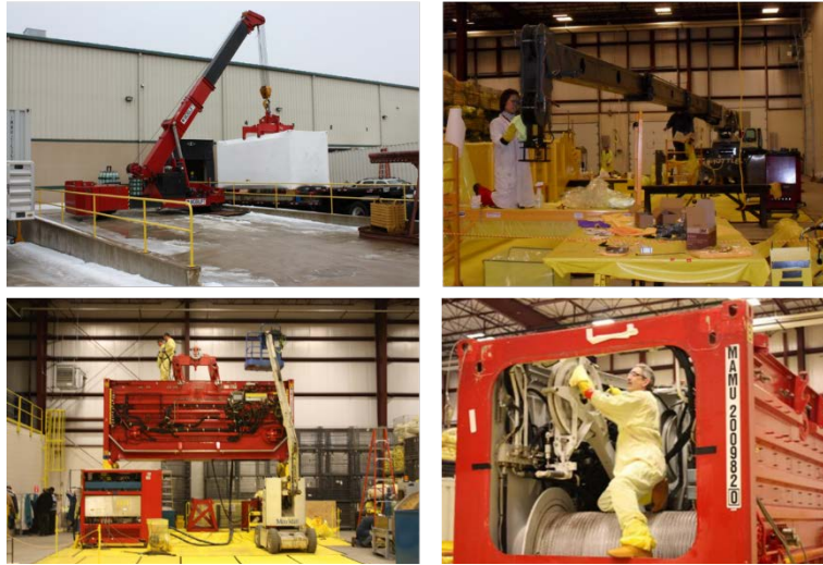
Figure 13 SG Replacement Crane
