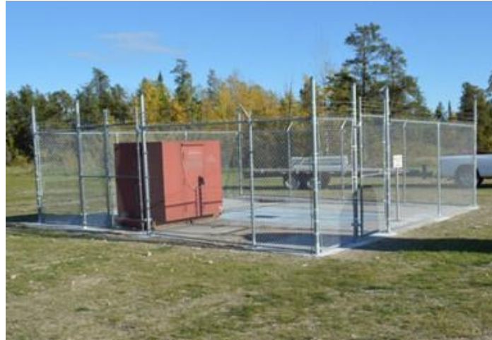
Figure 2 The monitoring enclosure near the main access shaft
