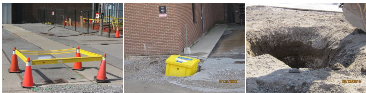
Figure 8 (a) catch basin sinkholes (b) buried service failure (c) yard drainage sinkhole uncovered
