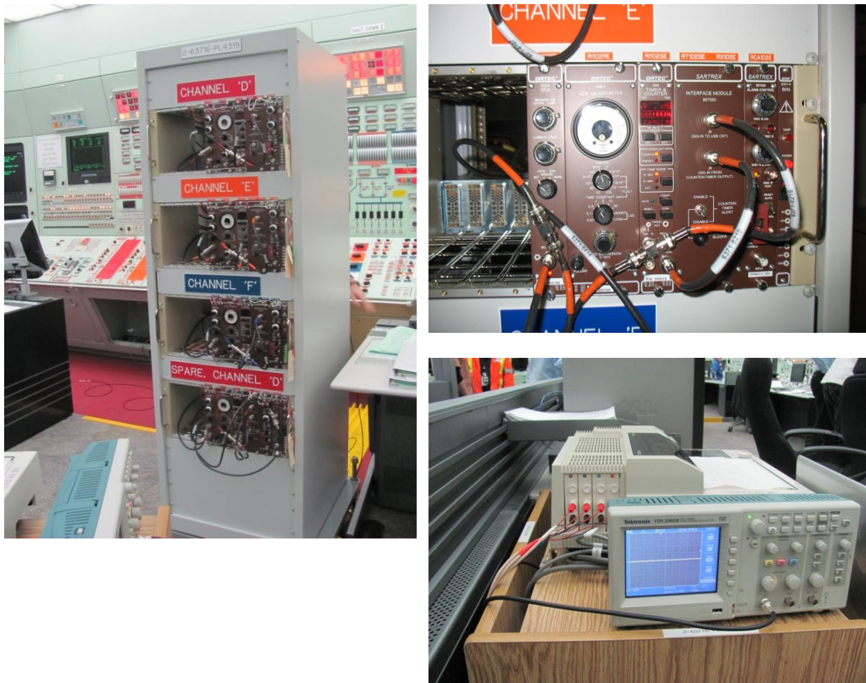
Figure 3 Start-Up Instrumentation in Main Control Room
