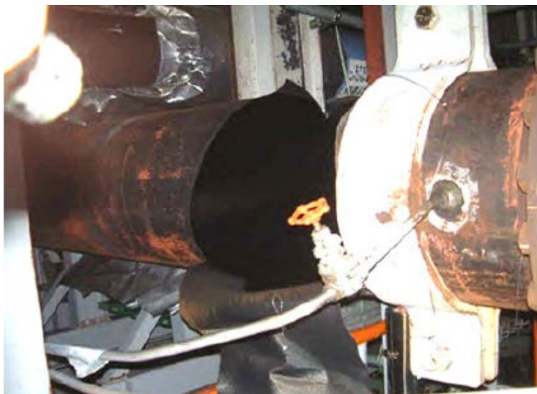
Figure 2 Ruptured Condensate Pipe at Mihama Unit 3(W. H. Ahmed [8])
