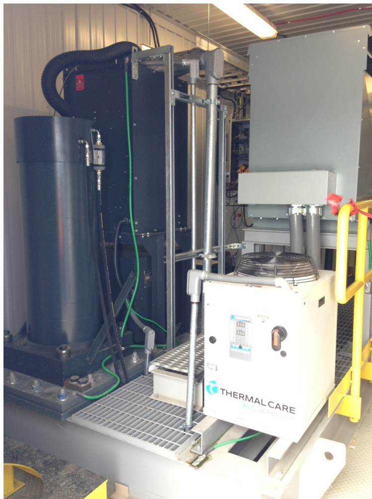
Figure 7: Flywheel Energy Storage System
