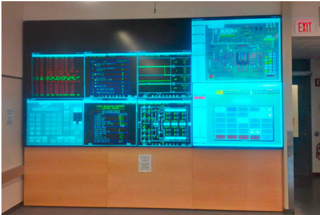
Figure 3 Use of six back-projection units showing multiple control room displays
