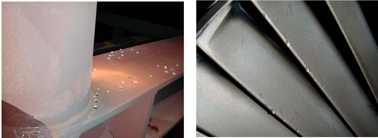
Figure 5. Condenser (left) and feed water pump steam turbine (right)
