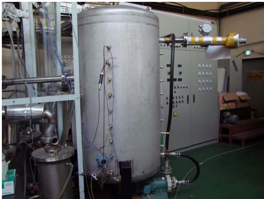
Figure 3 Installed storage tank
