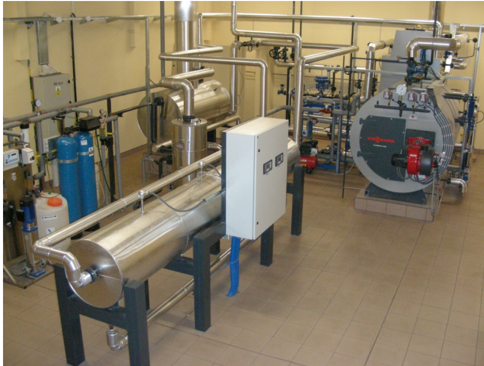
Figure 4 View of the experimental installation for testing the computer system for on-line monitoring thick-wall pressure components
