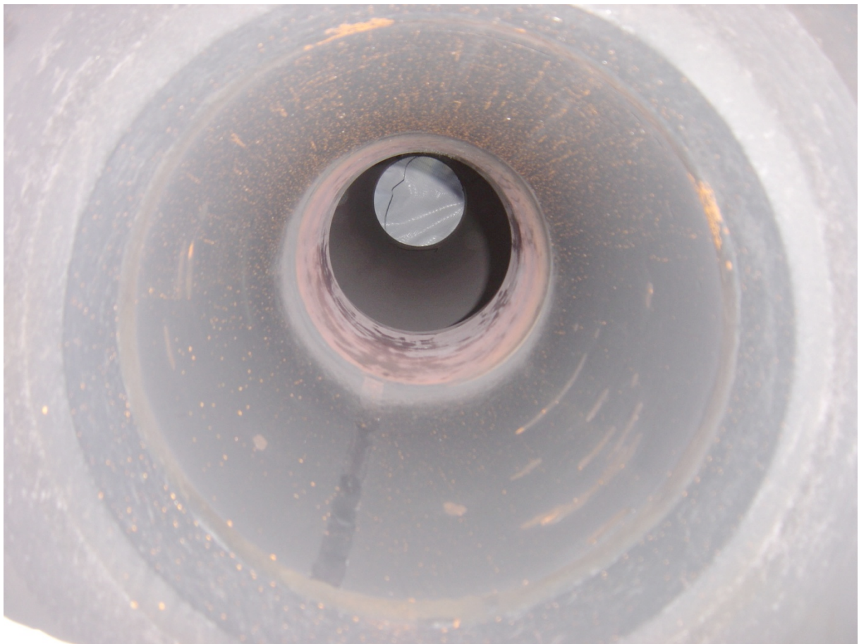
Figure 4 Photo of venturi meter viewed from diffuser end
