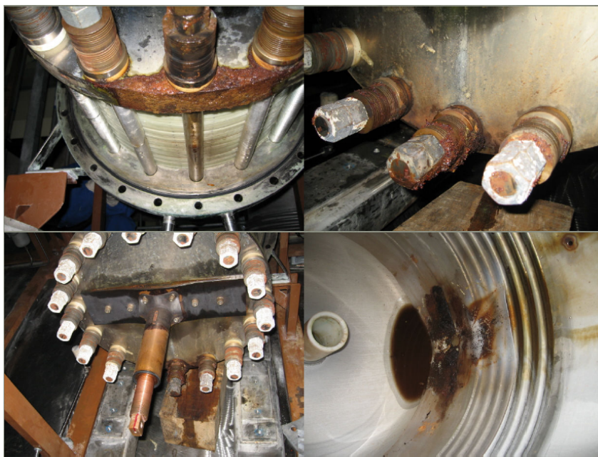
Figure 4. Corrosion in an Alkaline Electrolyser which is caused by caustic entrainment.
