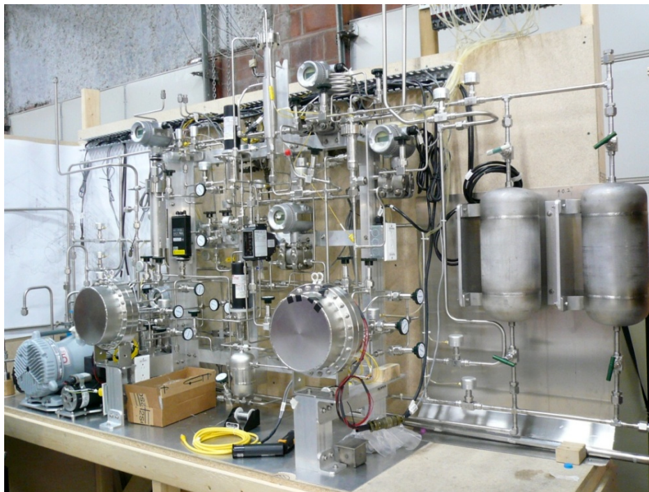
Figure 5. a mini CECE process rig for testing membrane in radioactive environment.
