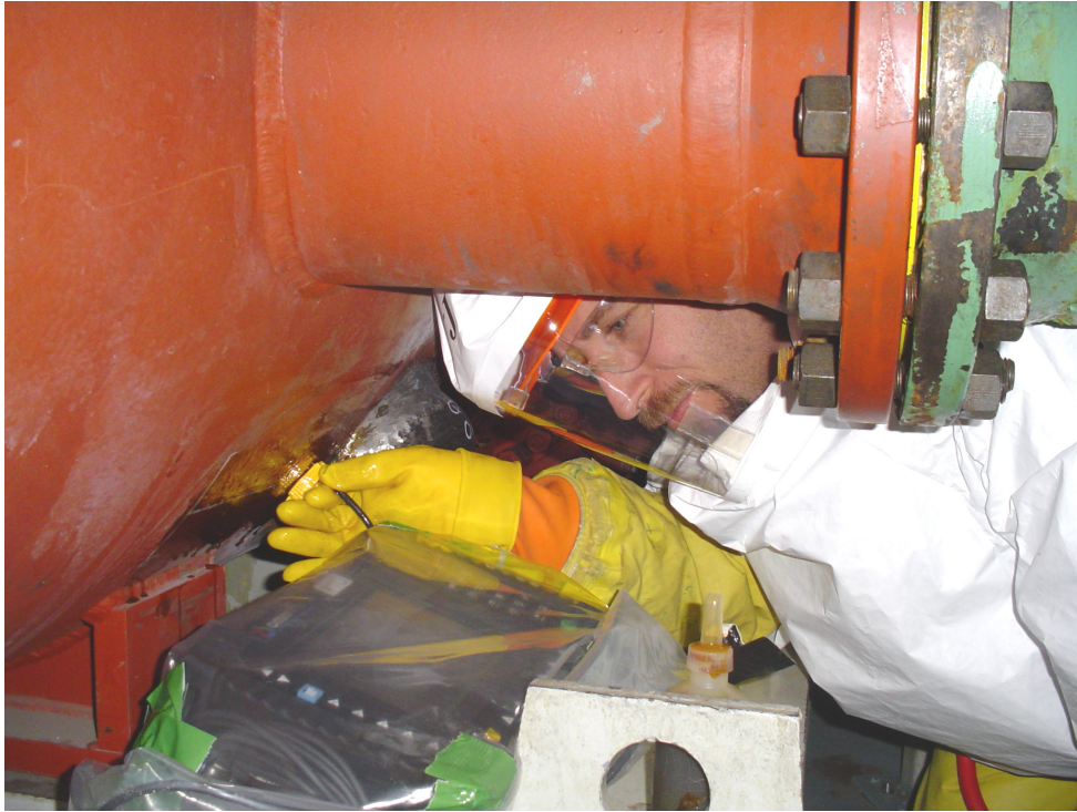
Figure 8: Example of PAUT inspection of SDC- HX with L-waves - PNGS U4.
