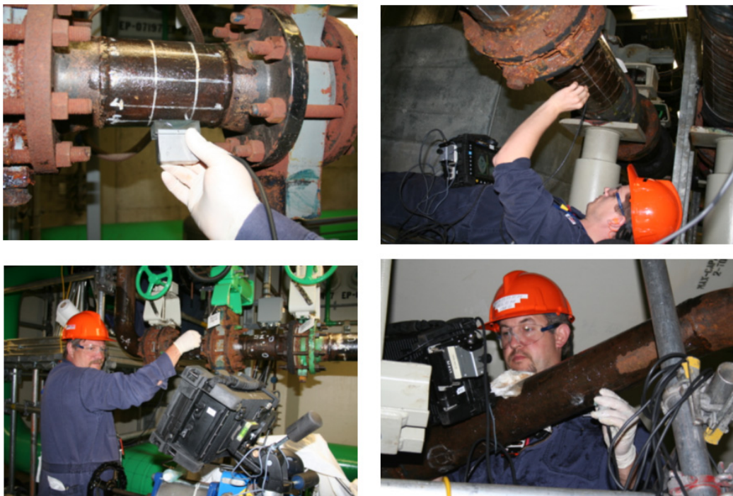
Figure 11: Examples of field inspection of secondary service water lines at DNGS.
