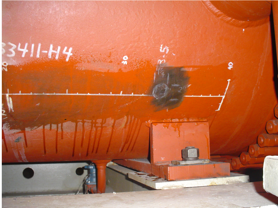
Figure 10: MIC attack location in HAZ of lower weld on HX 4.
