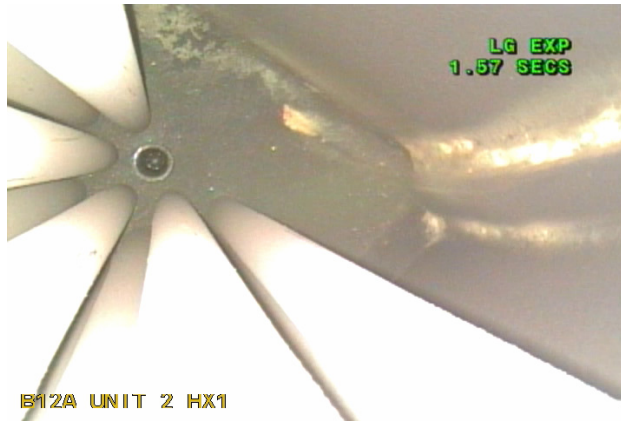
Figure 7 – Preheater Secondary Side (Tubes, Baffle Plate, Shroud and Divider Plate)
