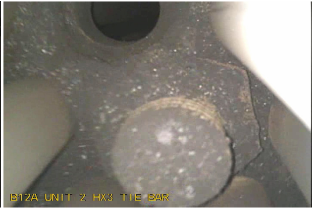
Figure 6 – Preheater Secondary Side (Tie Rod Location on Baffle Plate)
