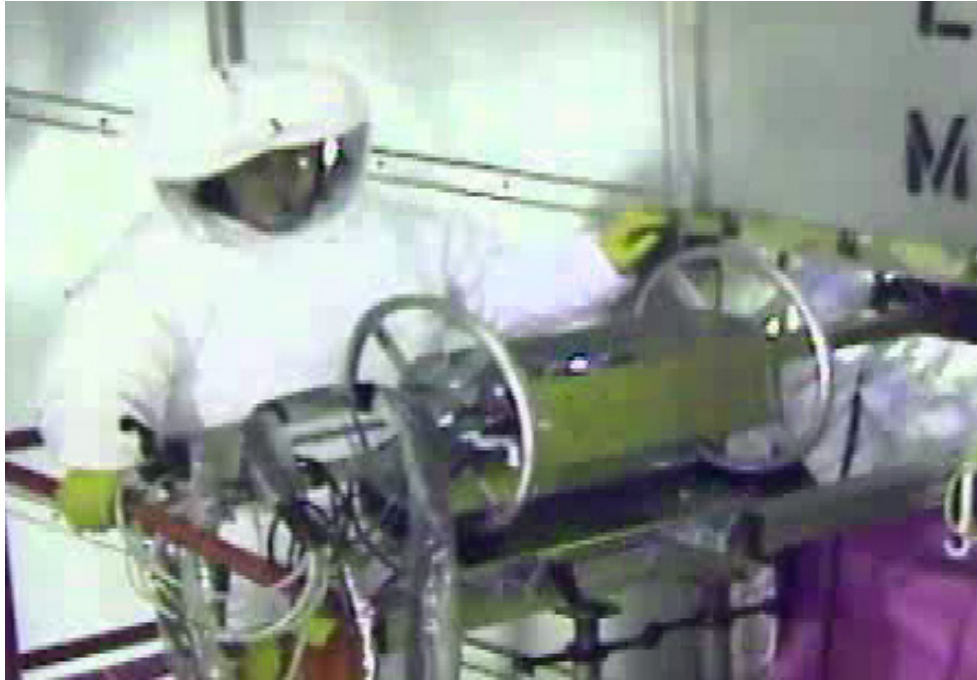
Figure 8 – Weld Head (installed on-reactor)
