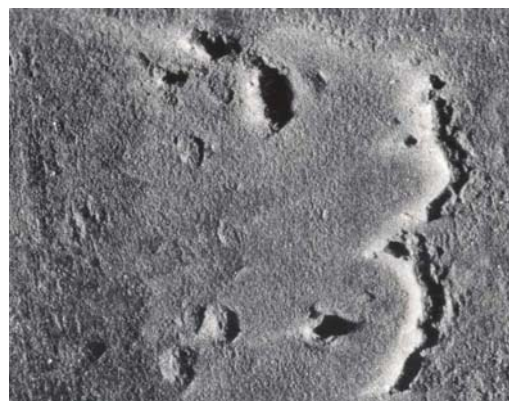
Close-up view of the affected region
