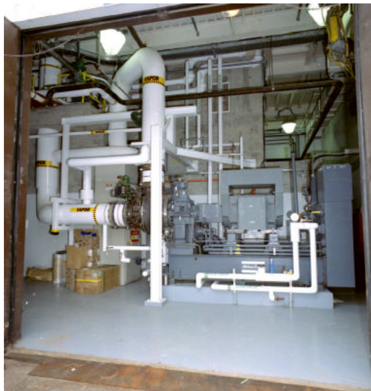
Figure 4. LWE Vapour Compressor
