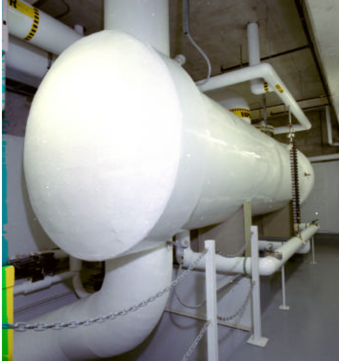
Figure 2. Main Heat Exchanger
