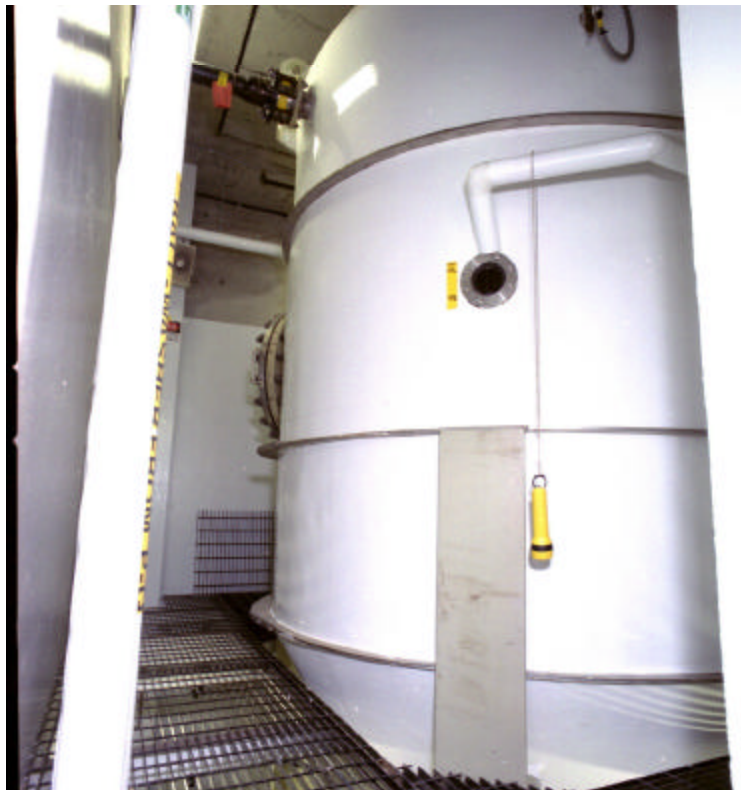
Figure 3. LWE Entrainment Separator
