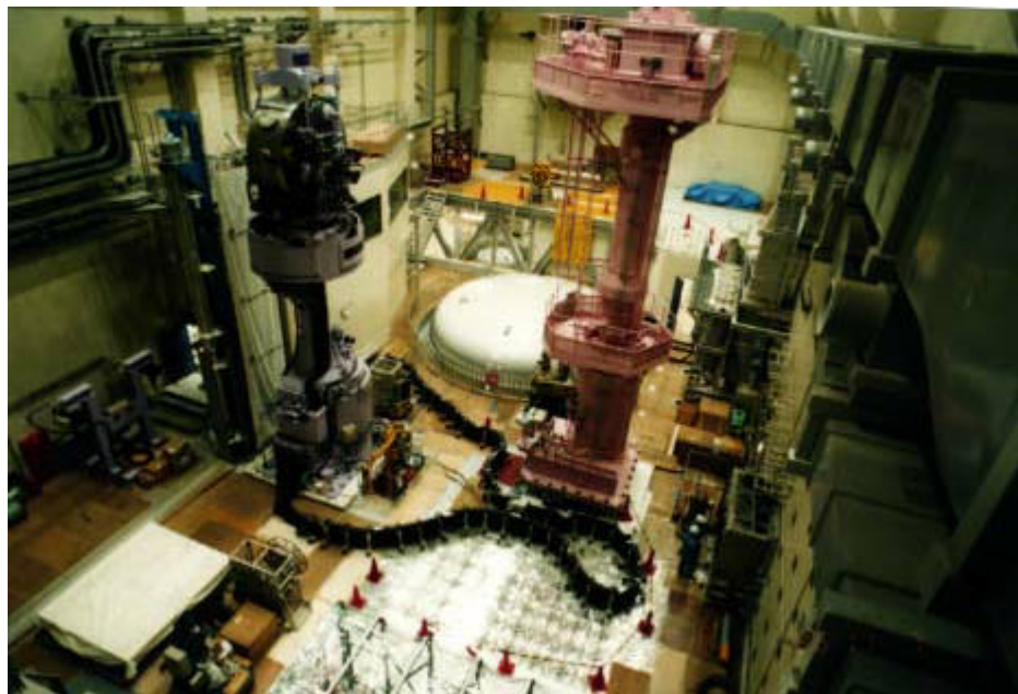
Photo 2 HTTR fuel handling area with fuel handling and control rod handling machines.
